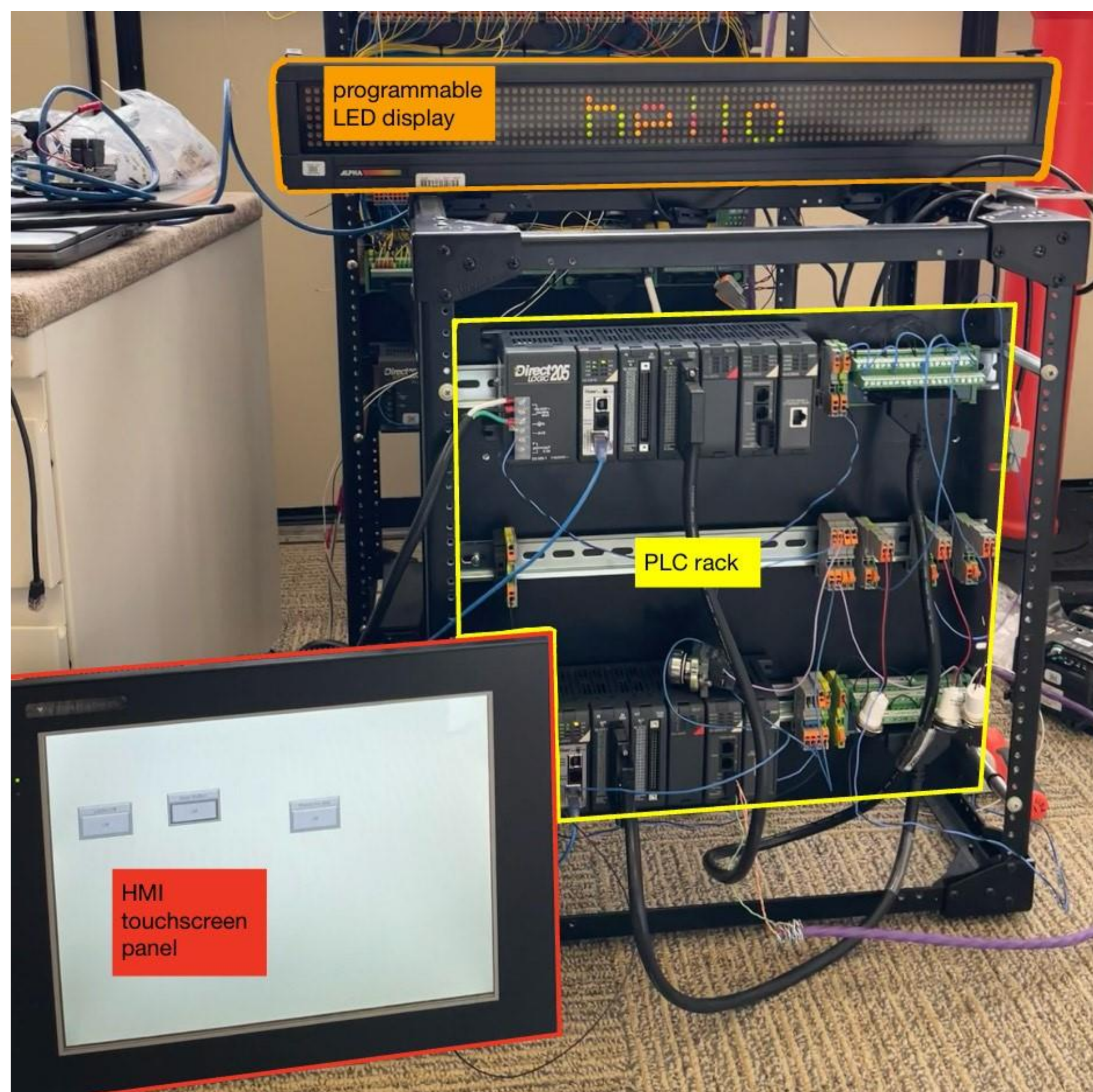
2-PLC system connected to HMI touchscreen and LED display via Ethernet
