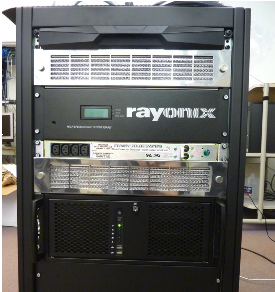
Figure 15 – MX225-HS Controller Cabinet front view
