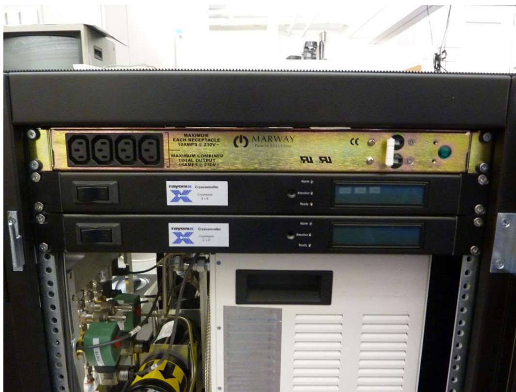
Figure 16 - Cooler Cabinet power switches
